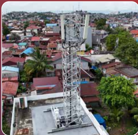
Figure 34. Glass Fiber Reinforced Polymer Tower
